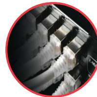
Copper Cabling & Connectivity
